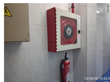
Fire fighting equipment.jpg
